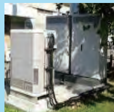
Base Station Equipment
