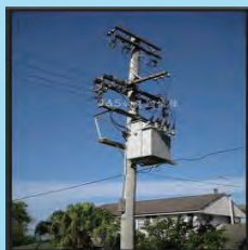
Outdoor Electric Equipment
