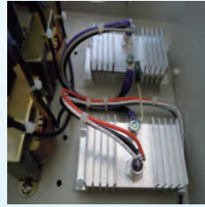
Stable Main Control Components
